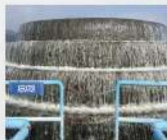
Aerator at Sri Gading Water Treatment Plant
